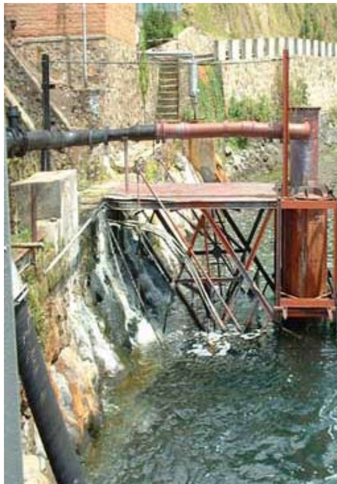
Demonstration of the methane exploitation for fuel use: A gas pipeline on Cape Rubona used by the Bralirwa Brewery
